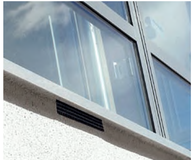
An example of concealed air intake below the window ledge flashing
